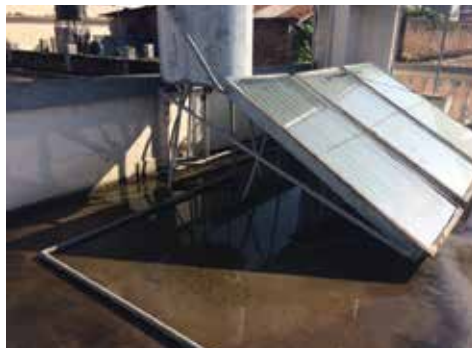
Roof top rain water collection under house solar panel
